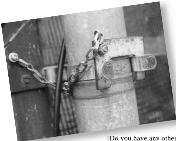
Home-made steel U-clips prevent the wind from springing the mast out of the Terry clips that hold it up.
