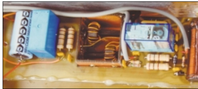
T1 and T2 can be seen clearly inside the SWR head. In this view, RL21 is to the left of it and RL20 is to the right.
