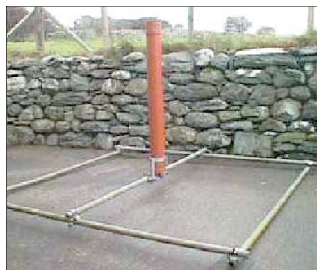
The GB3GW aerial mounted on its support frame prior to installation.
