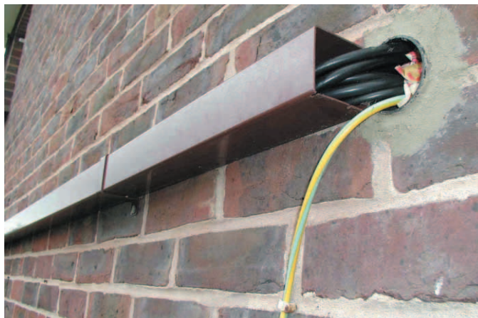
The arrangement for routing coax and other cables from inside the shack at the front of the house to the rear. There is plenty of room for future additional cables. The yellow cable is a safety earth wire connected to ground.
