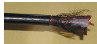
The rogue coax length. The centre conductor is nice shiny copper although the braiding is a dull black colour.
