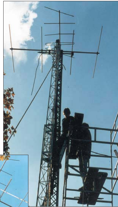
John Eley, G3LMR, replacing the tower carrying his 6m 4-ele, 2m 5-ele and 70cm 8-ele Yagis. John says that the old tower (right) was installed 20 years ago but had rusted through at the base. In the photo (left) the new tower is being used as a crane to lower sections of the old tower to the ground.
