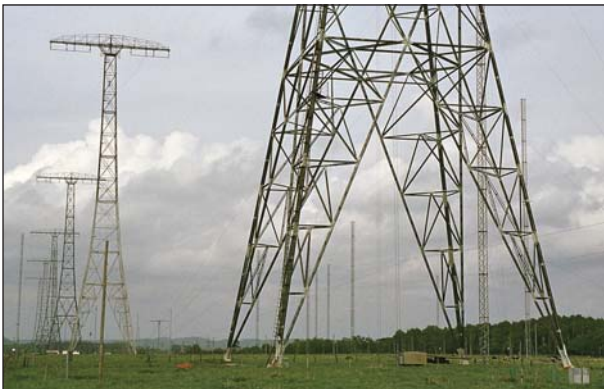
The 2200m-long multiple tuned antenna is an eye-catcher from the Swedish west coast railway and the E6 motorway.
