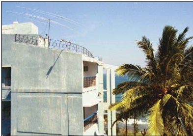
The antenna support was bent during the earthquake.
