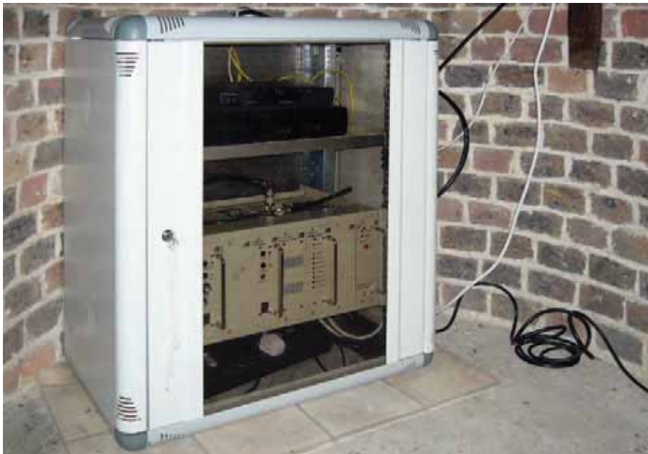
The homebrew D-Star node lives in a professional-looking rack enclosure in the tower of St. Leonard's Church, Turners Hill.
