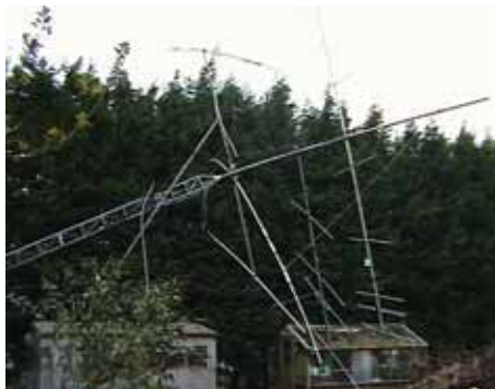
The winds can be high in Wolds, the site is completely unshielded to storms coming in off of the North Sea!
