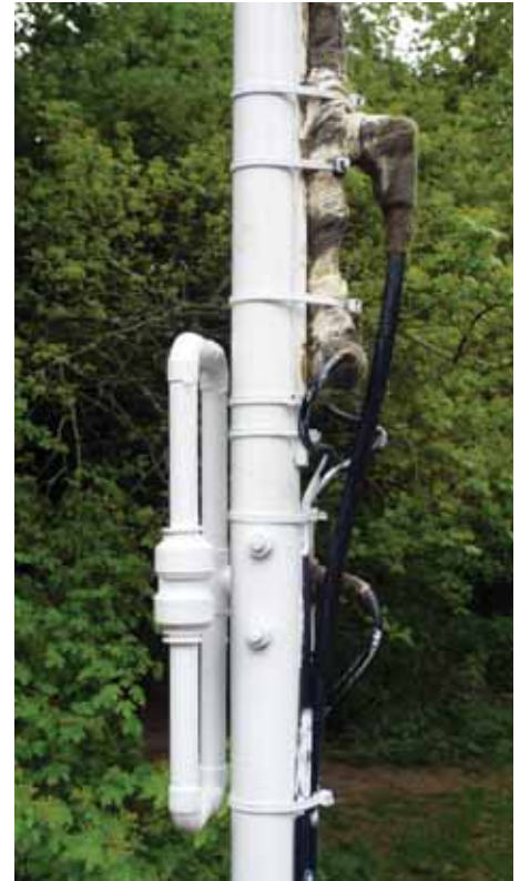
PHOTO 5: A completed dipole mounted on the pole with part of the power splitter on the right.
