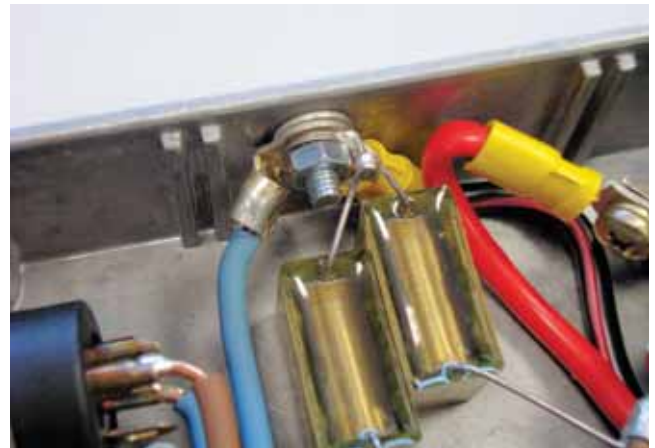
PHOTO 3: Common earthing point using solder tags for different connections.
