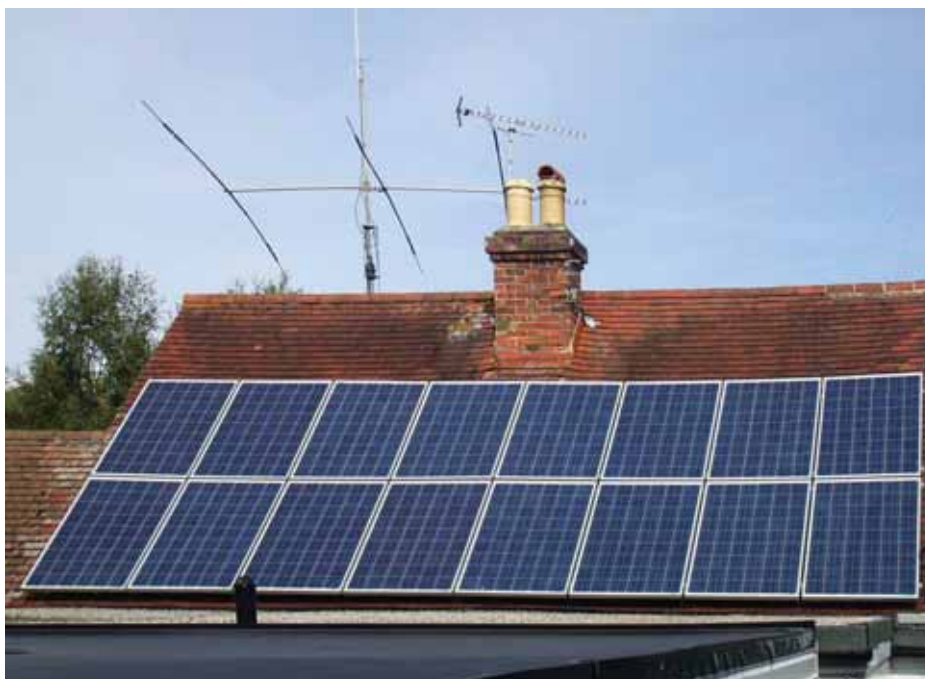
PHOTO 2: Photovoltaic micro-generation system at G4CUS.
