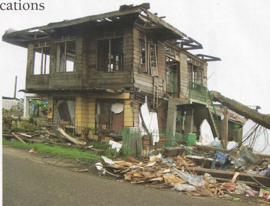
Badly damaged house near Tacloban City.
