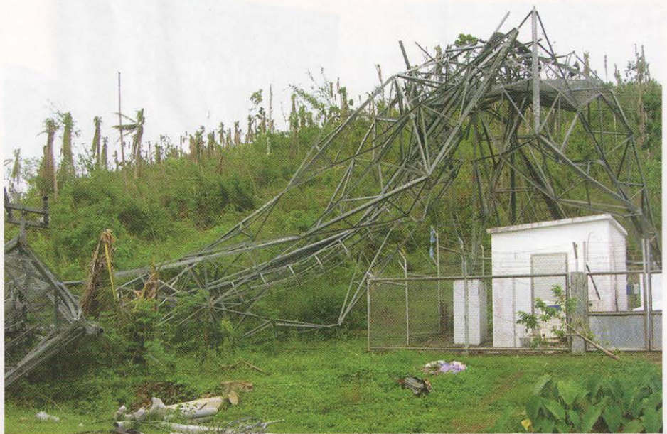
Collapsed 3G mobile phone mast 50km south of Borongan.
