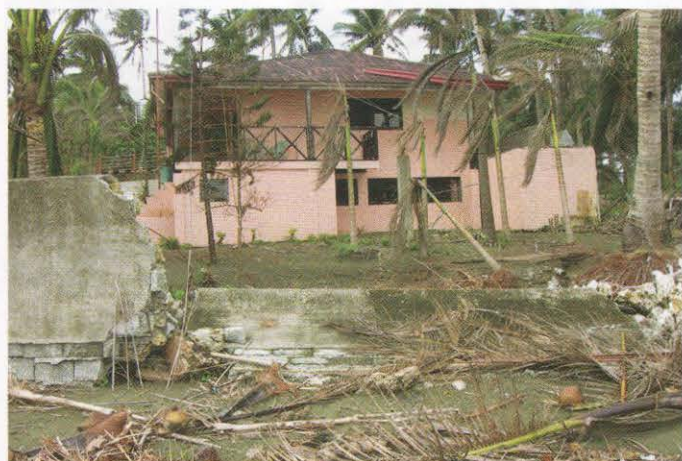
Breached sea wall at DV5PO.
