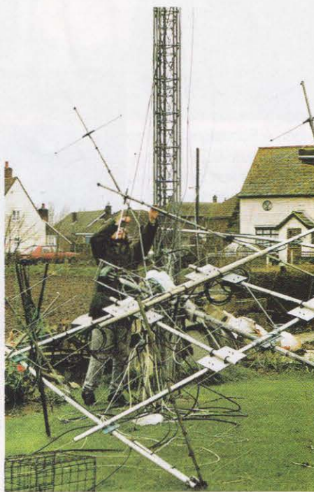
The amateur's worst nightmare - a blown-over tower.
