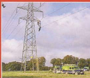
Cover image: SEPD engineers replacing suspect insulators on a 132kV power line. Photo: Brian Coleman, G4NNS.
