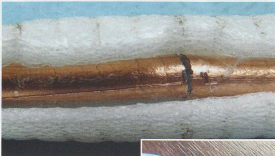
PHOTO 1: A break found in the centre conductor of a piece of Superflex coax by Mike, GOMJW.
