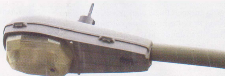
PHOTO 1: A typical modern street light with an antenna (top) for remote control and monitoring.
