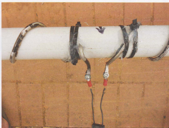
PHOTO 3: Helically-wound loop open-wire line feedpoint before silicone sealant was applied to the stainless steel hardware electrical connections.
