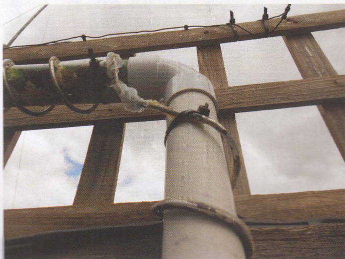
PHOTO 2: Silicone sealant coated aluminium wire joint (one of four).
