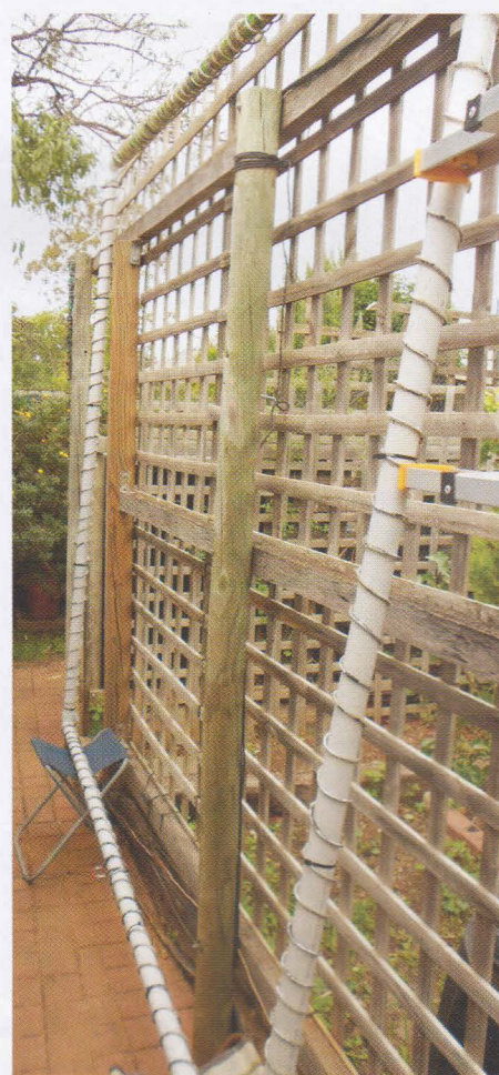
PHOTO 4: Frame Loop aerial raised & leaning against trellis during silicone sealant curing period.
