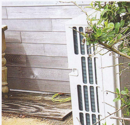
PHOTO 1: Non-standard earth wiring (green/yellow coil of wire) associated with an air source heat pump (ASHP).
