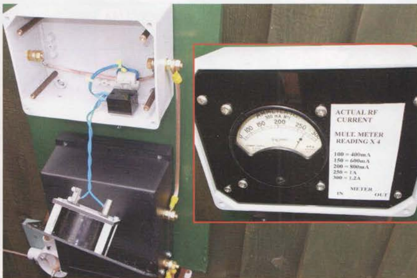
PHOTO 8: The RF ammeter and (inset) front panel. Inside the box the black item connected to the blue wires is the on/off switch; the white item behind it is the 2:1 current transformer core.
