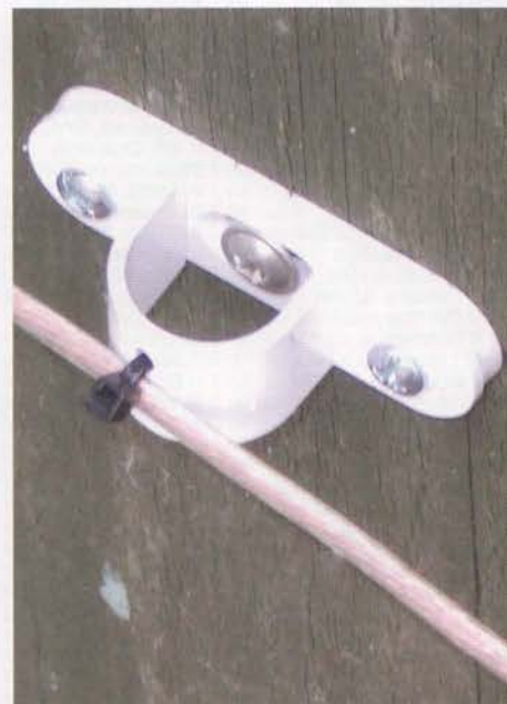
PHOTO 2: Wire attached to saddle clamp. Note how I used a cable tie to attach the wire to the top of the clamp, rather than mounting the clamp vertically and letting the wire run freely through the saddle, as this arrangement makes it easier to stop the wire sagging.
