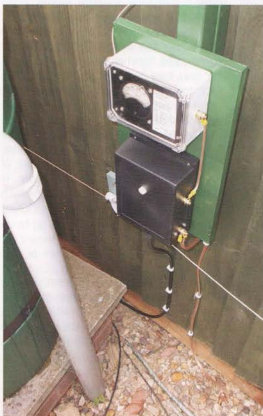
PHOTO 7: The transformer in situ, with the RF ammeter above. The earth spike is at the bottom right of the photo.
