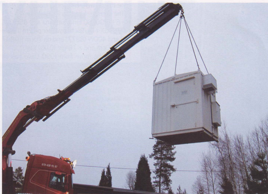
The remote shack installation for Anders, SM4KYN in Sweden.
