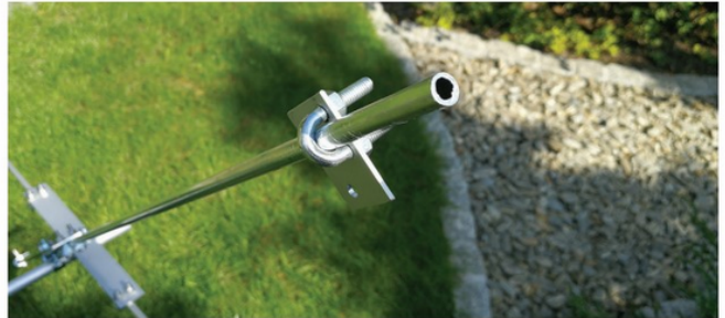
PHOTO 7: A small aluminium plate and a galvanised steel clamp create a corner of the end frame. Do not forget to use Cu-Al washers in all spots where copper wire would touch aluminium plate or tube. Also be aware that the clamps may degrade over time.
