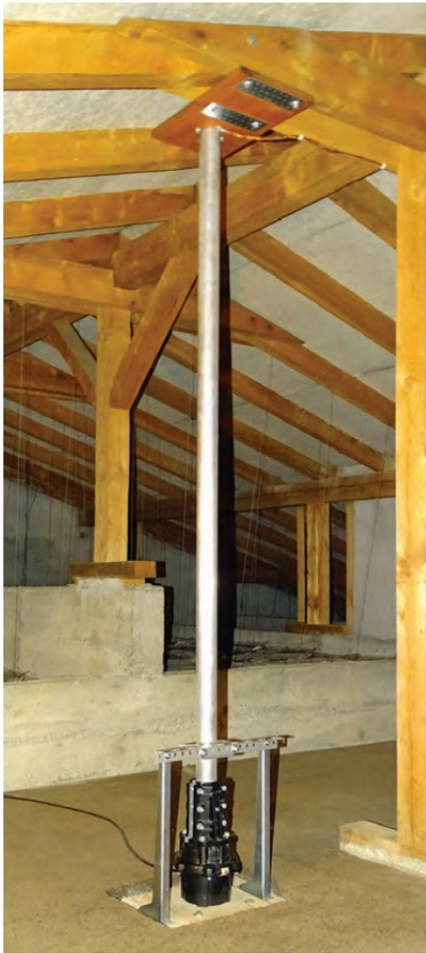
PHOTO 3: Mast base with rotator in the attic.
