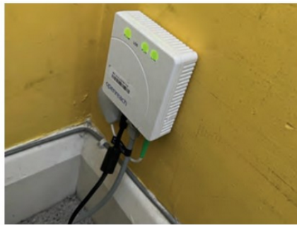
PHOTO 1: A typical Optical Network Terminator (ONT) for Fibre to the Premises (FTTP).
