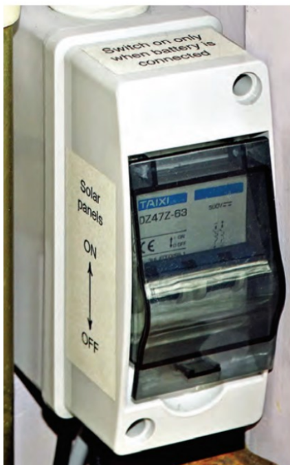
PHOTO 6: A DC circuit breaker is required to isolate the solar panels from the charge controller.
