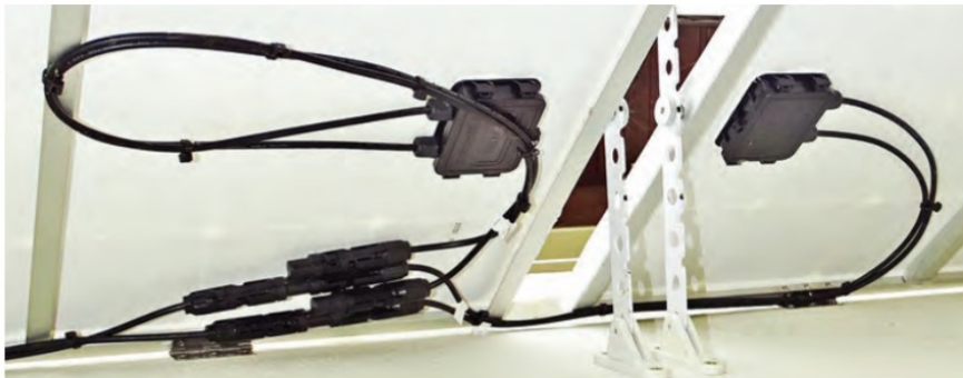
PHOTO 3: Parallel interconnection of two solar panels with MC4 adaptors.
