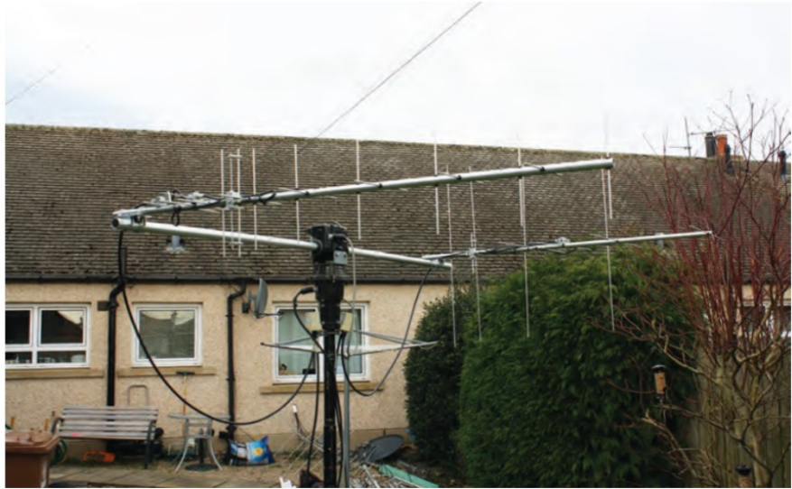
The finished installation, complete with azimuth/elevation rotator.
