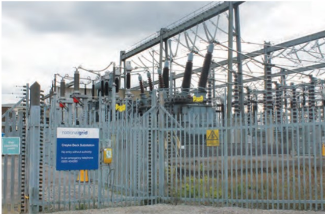
PHOTO 1. A typical 400kV National Grid substation.
