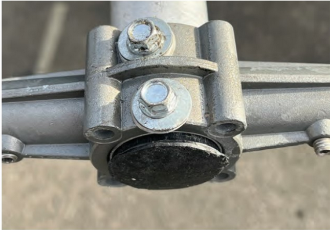
PHOTO 3: Not the original screws here.
