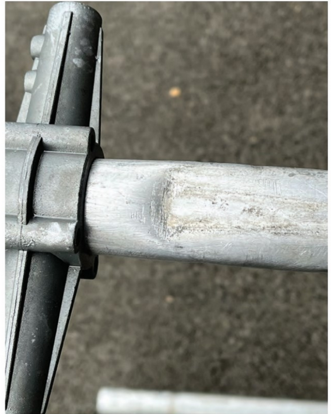
PHOTO 2: Over tightening of the mast clamps causes tube malformation.
