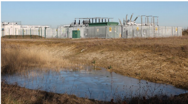
PHOTO 1: The Pelham Battery Energy Storage System.
