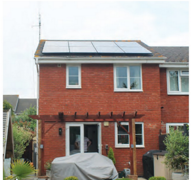
PHOTO 1: A recent solar PV installation with outdoor ground-mounted inverter.
