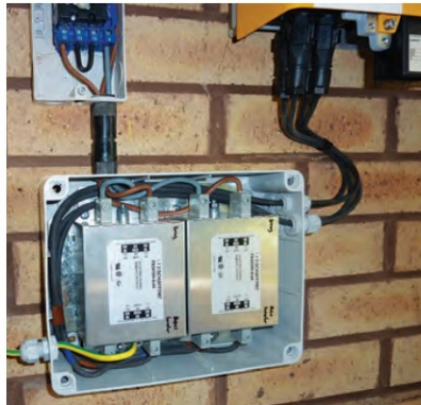
PHOTO 1: Two Schaffner FN2410H-8-44 filters fitted to the DC inputs of a solar PV system.
