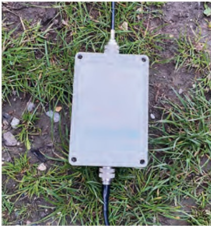
FIGURE 3: The line isolator attached in line with the RG-58 coaxial cable.
