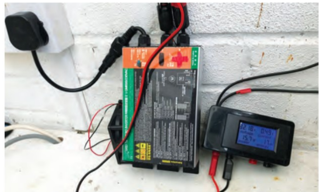
FIGURE 4: Grid-tied micro inverter, and the combined current /voltage monitor used to measure the solar panel's input. A fan has been added to keep the unit cool when running at full power in a hot conservatory.
