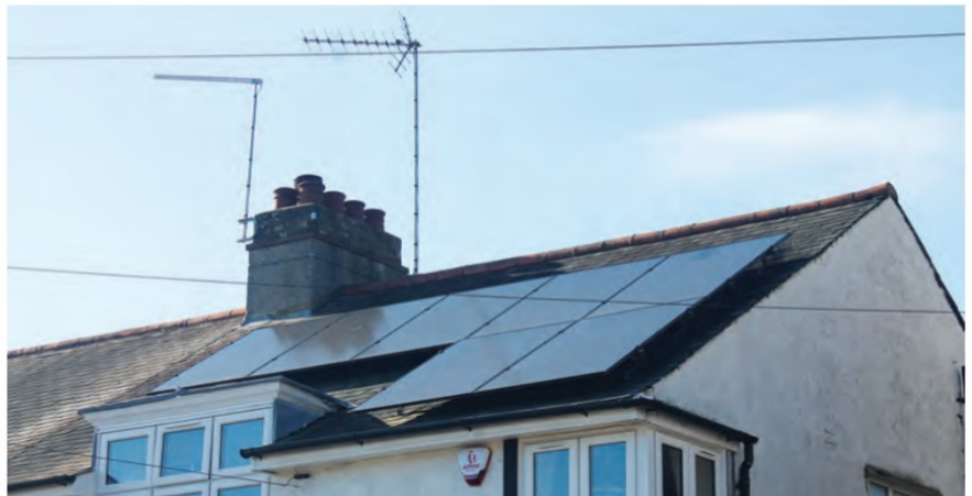
PHOTO 1: A typical solar PV installation.
