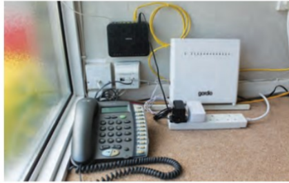
PHOTO 2: A full fibre broadband installation alongside a copper VDSL2 installation.
