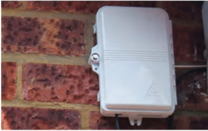
PHOTO 1: An outdoor Customer Splice Point (CSP) box.
