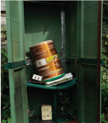
FIGURE 4: This shows what can happen when 700W at 137kHz is mishandled. Here, small spark gaps were created when overlapping metal tape was used to seal the plastic cabin joints. In the vicinity of the fields around the loading coil, sparking at the joints of the tape set fire to the plastic.
