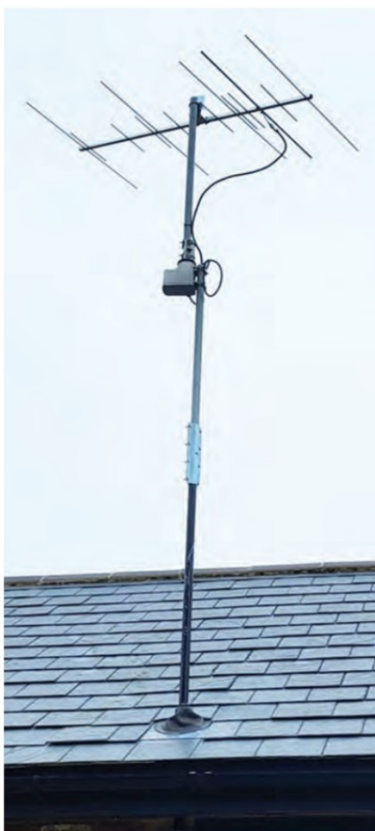
FIGURE 1: The antenna rotator mounted on a pole fixed to my roof.
