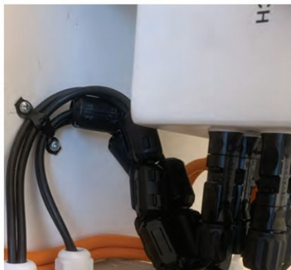
PHOTO 2: Clip-on ferrite cores fitted to a solar PV installations.
