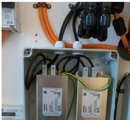
PHOTO 1: RF interference filters fitted to a solar PV installations.
