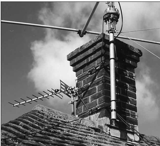
Fig 13.36: Example of a chimney lashing used to support a double-D antenna
