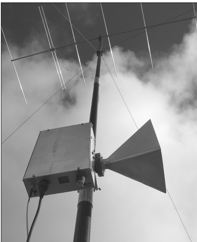
Fig 18.34: Transverter and horn mounted on the mast, aligned with the 2m talkback antenna
