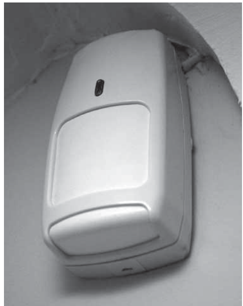
Some alarm PIR detectors are also prone to being triggered by stray RF.
